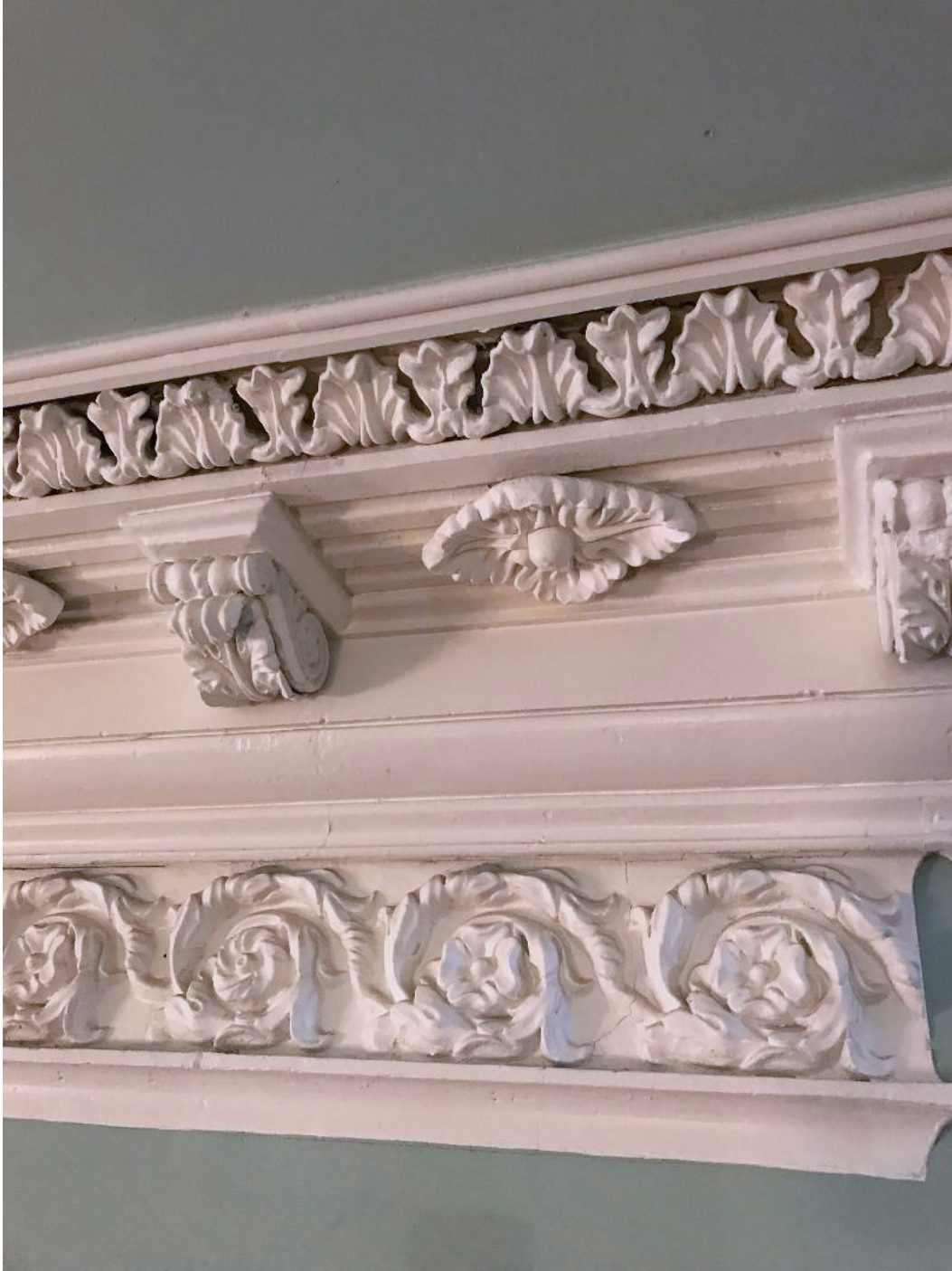
Extraordinary original plaster molding in the central hall. Photo courtesy of Peter W. Patout April 2018.
